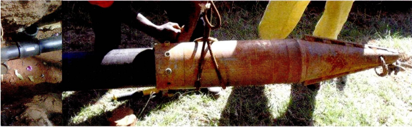
ABOVE FROM LEFT Bursting asbestos cement pipes, 60 t rod puller, pipe-bursting steel pipe, T135 Hammer in 160 HDPE bursting casing
