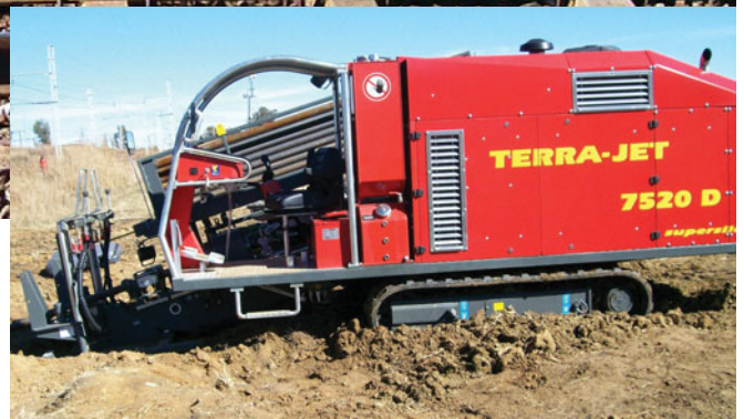
TOP The railway line near Sasolburg ABOVE The TERRA-JET 7520 D during the 40 m-long pilot bore underneath the railway tracks
