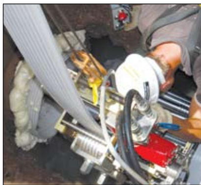
Formed pipe being progressively fed to the right, into existing concrete pipe. Note previously completed section on the left
