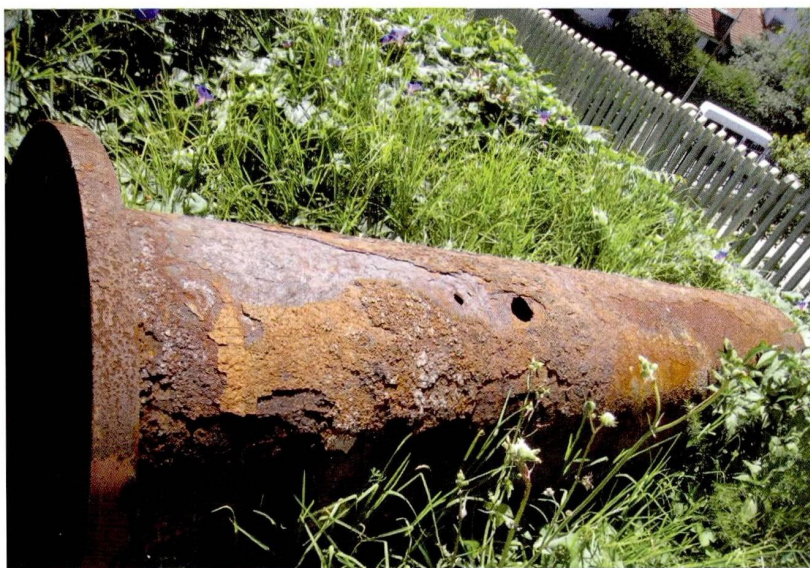
LEFT Sample of a removed corroded section of 600 mm steel pipe
